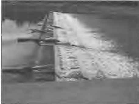
The Island Farm Weir in New Jersey featured a dangerous reverse roller (above, Bruce Tschantz), until a baffled fish ladder was retrofitted in 2013 (below, Paul Schweiger).
