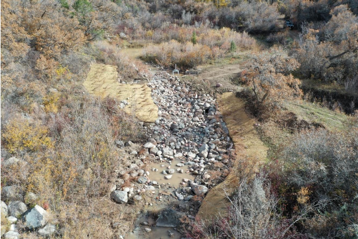
Aerial view after construction (November 2021). Photo credit Scott Schreiber, Wright Water Engineers.
