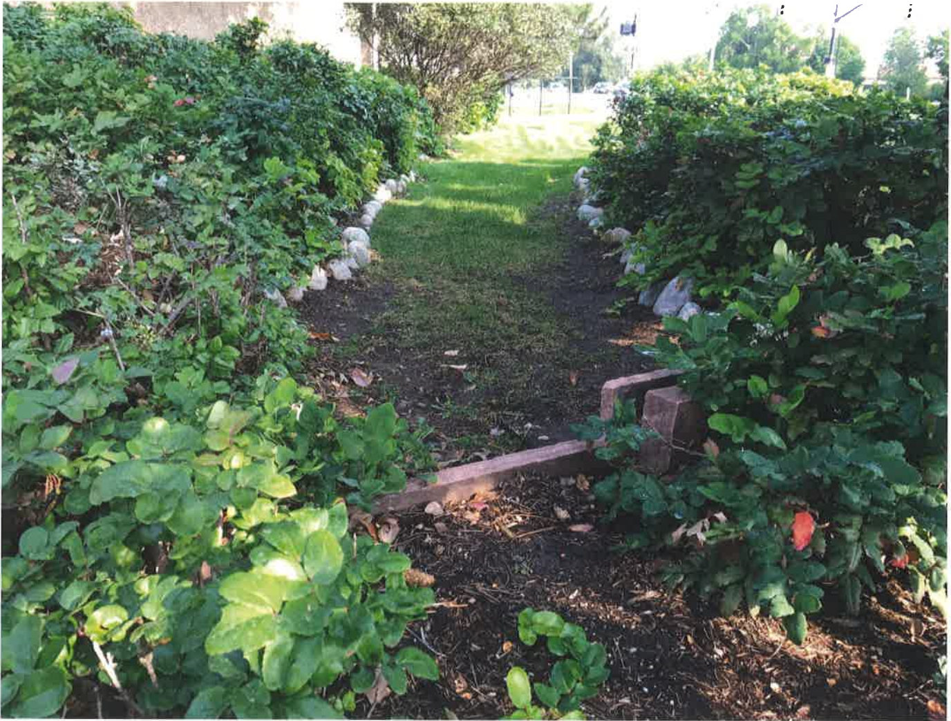
Figure 7. One of three water storage check dams/weir structures installed on the east perimeter of the WRA property to increase onsite stormwater capture volume. Date: 2017.
