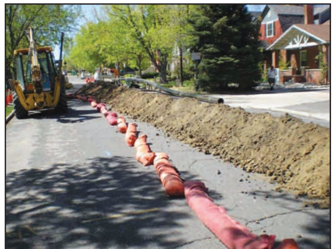
Rock socks at street crown confine temporary stockpiles to one side of street.
